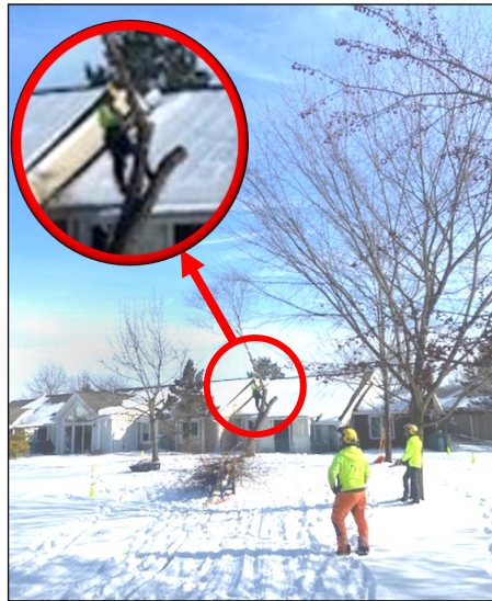
Birch behind Cottage 104 being taken down. Notice worker up in the tree. Photo credit: Tree Contractor
